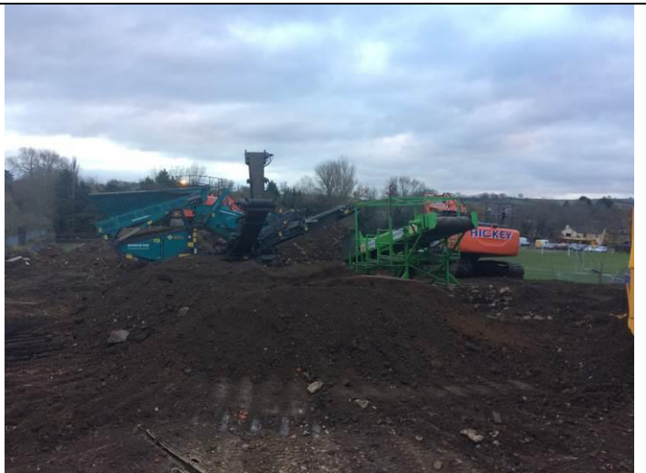
Photo 4: End of day (Wednesday 29.11.17) after beginning of removal of material off site.
