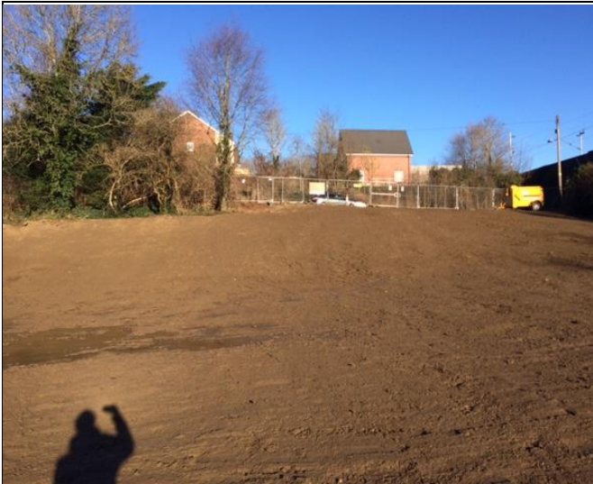
Photo 1. View of the site showing off the levelled ground leading up to Bridge Street.
